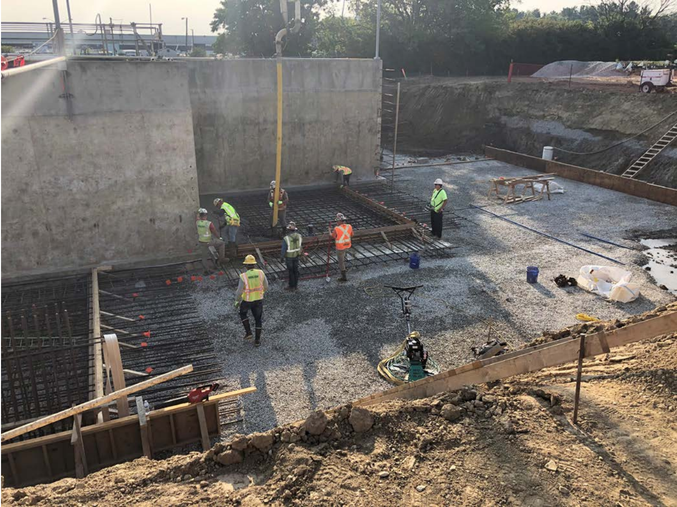
Economic growth in McCordsville has caused the need to expand the Wastewater Treatment Plant facility. This expansion should be completed in late 2021.
